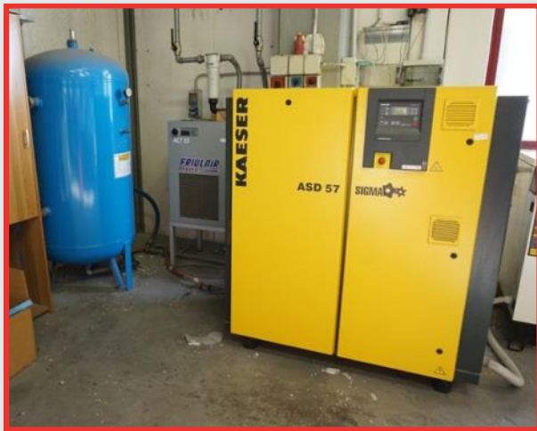
• Kaeser ASD57 Compressor plus other Compressors
